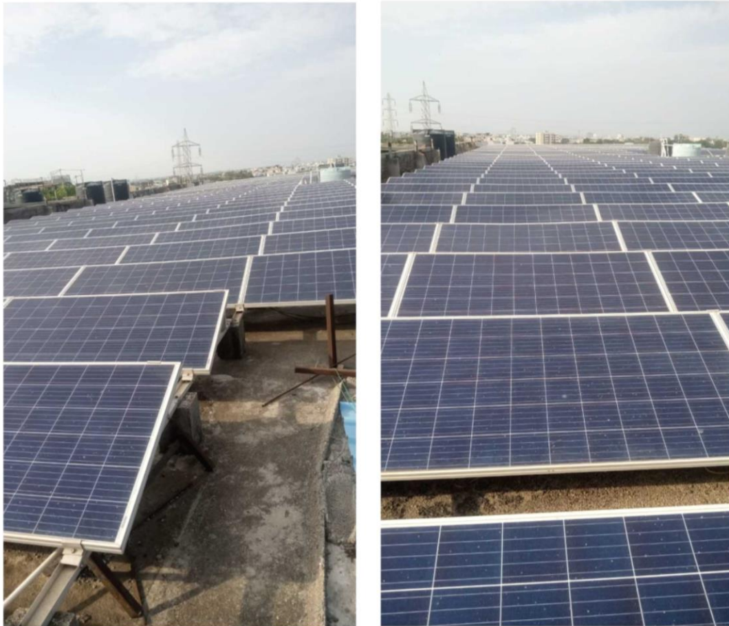
Rooftop Solar System with 110 KW Capacity
